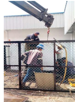
Repair Works – Transformer And Other Rectification Works At Lot 10, Jalan Tandang Petaling Jaya (Sapura@jalan Tandang)
