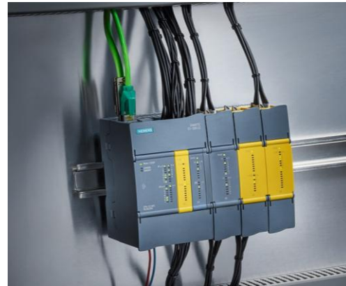
Data Acquisition: Siemens S7-1200 G2 Controller capturing real-time machine signals.
