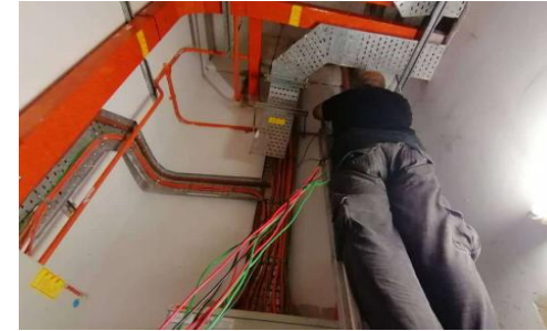
Kerja – kerja Pembaikan Closed Circuit Television (CCTV) Di Institut Latihan Kementerian Kesihatan Malaysia Sungai Buloh, Selangor.
