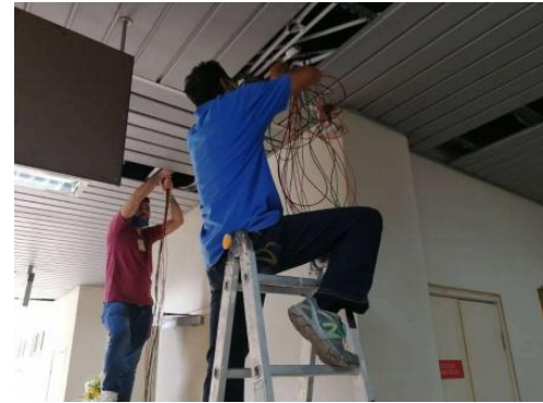
Kerja – kerja Pembaikan Closed Circuit Television (CCTV) Di Institut Latihan Kementerian Kesihatan Malaysia Sungai Buloh, Selangor.
