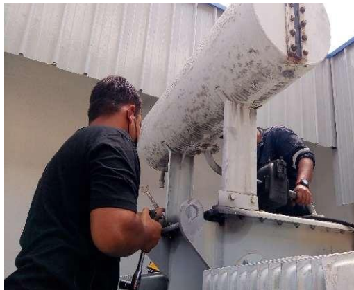
Repair Works – Transformer And Other Rectification Works At Lot 10, Jalan Tandang Petaling Jaya (Sapura@jalan Tandang)
