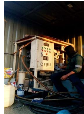
Repair Works – Transformer And Other Rectification Works At Lot 10, Jalan Tandang Petaling Jaya (Sapura@jalan Tandang)
